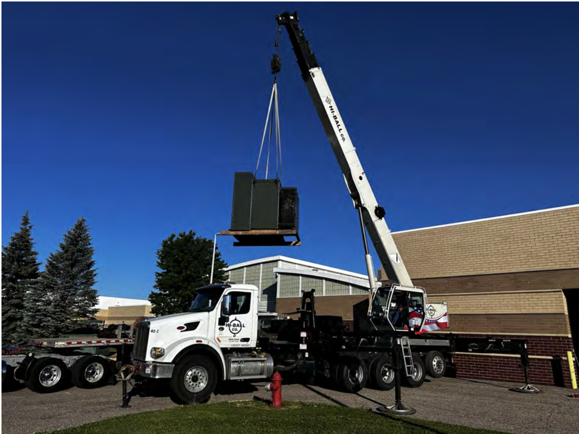
Pre-purchased high school transformer being delivered to the junior high for storage.
