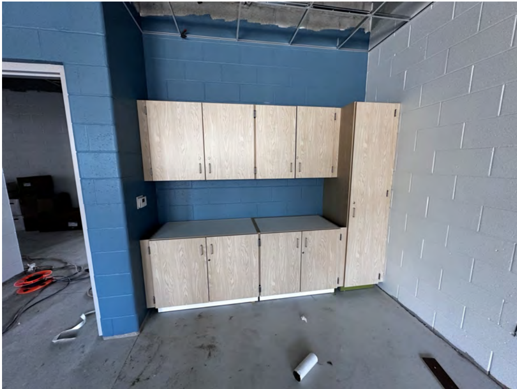
Classroom casework installed.
