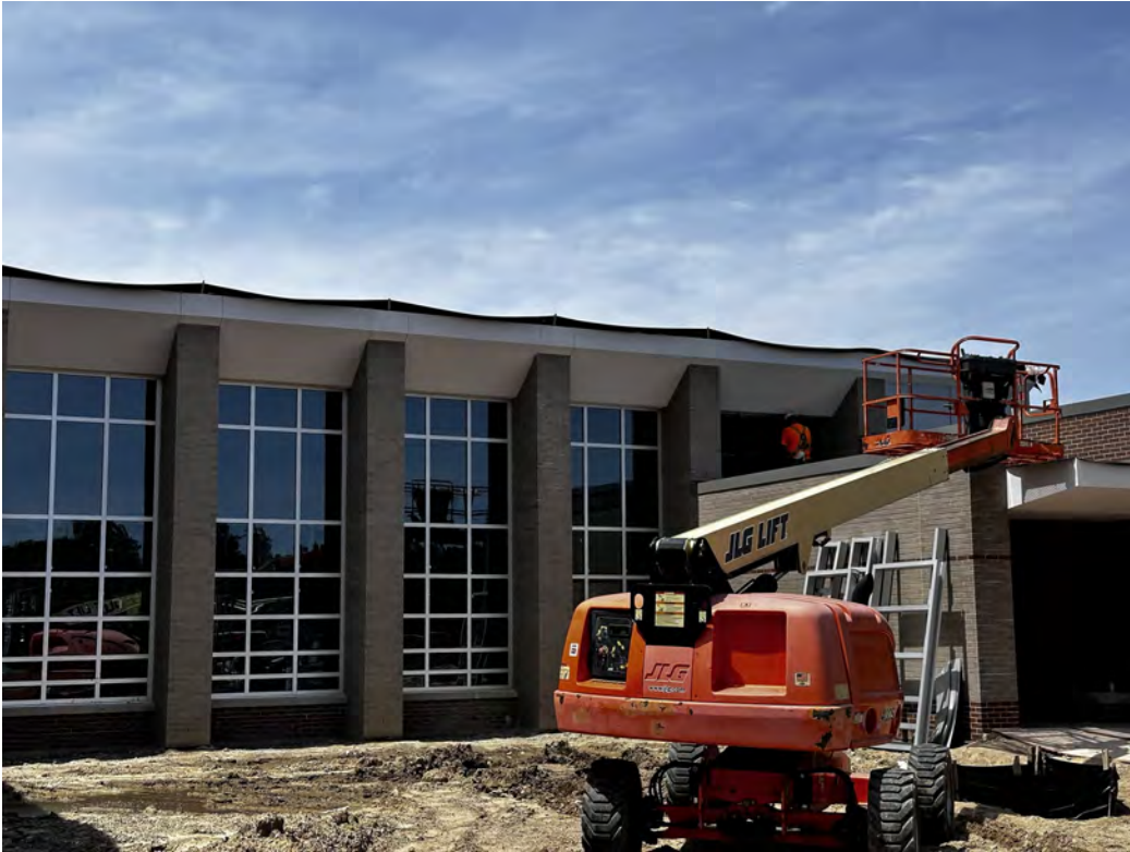
Direct applied finish system installed above curtain wall on east side of building.
