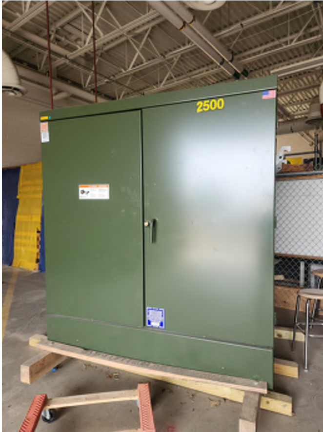
New transformer staged for install.
