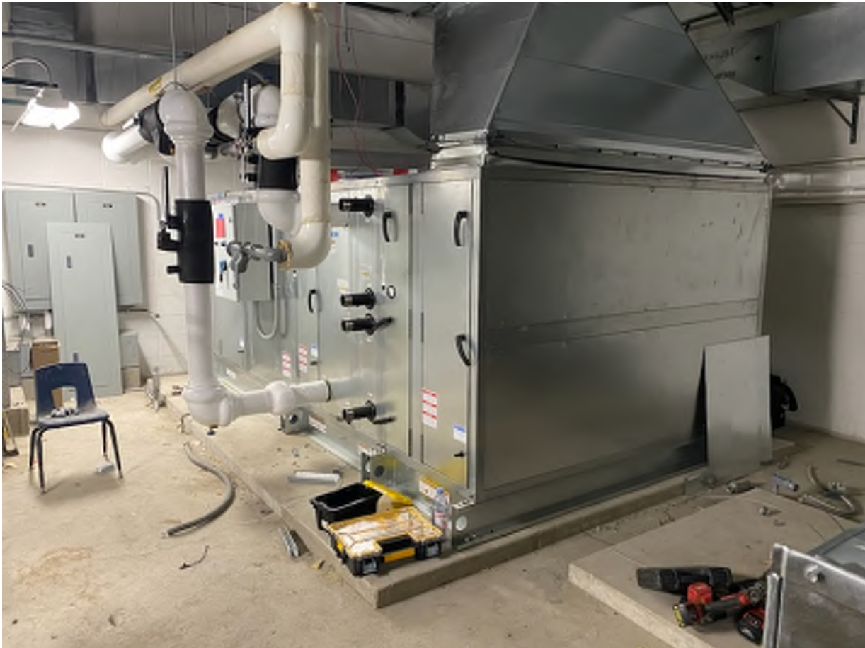
The new air handling unit in one of the three mezzanines.
