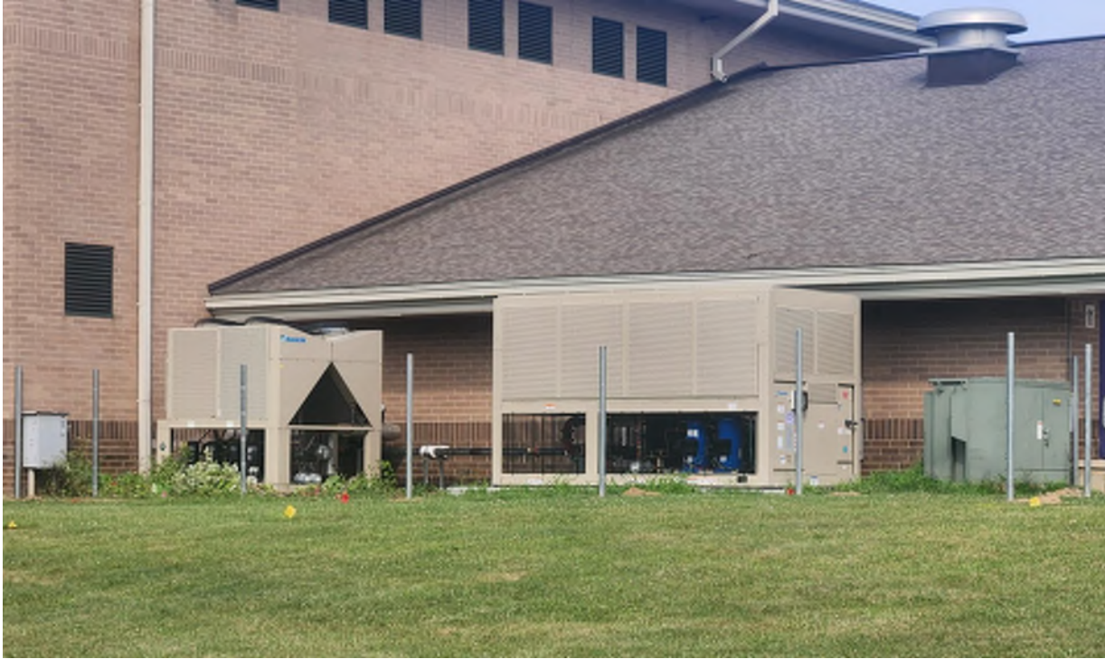
The chiller set on the east side of the building.
