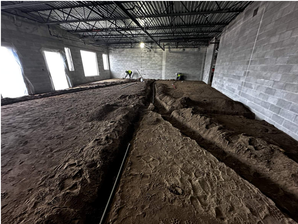
Electrical conduit installed in sand prior to concrete on east side of building.
