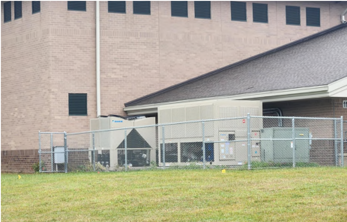
The chiller set on the east side of the building with fencing.
