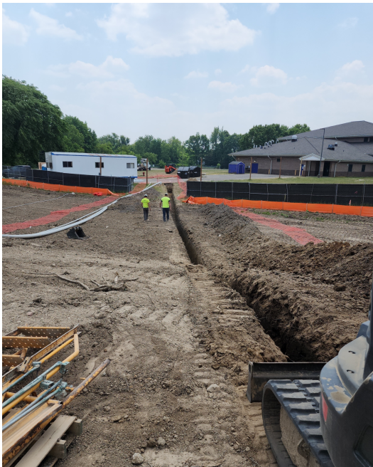
Boring for temporary power from Kreeger and permanent power for new building (complete).
