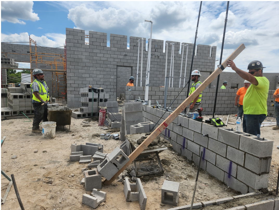
Plumbing and electrical trades working with masonry to coordinate in wall piping and conduit.
