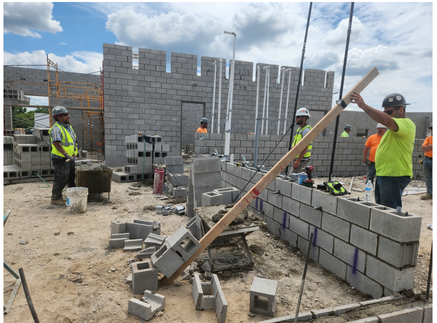
Plumbing and electrical trades working with masonry to coordinate in wall piping and conduit.
