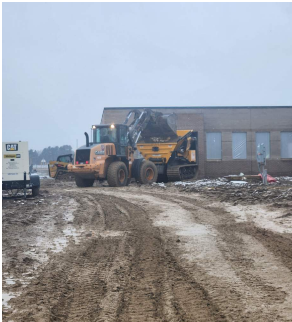
Sand being loaded into the slinger in order for it to be shot into building.
